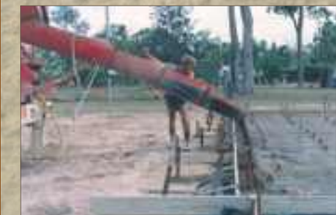
At left: Moisture is retained under the polythene membrane which in turn is a major attractant to Subterranean Termites
