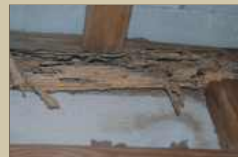
This Termite infestation is typical of homes constructed on a concrete slab, many within the first 12 months following construction.
